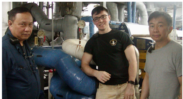
The Military Sealift Command fleet replenishment oiler USNS TIPPECANOE was recently honored with the Navy's Energy and Water Management Award at the Platinum Level. The ship's Chief Engineer Sam Battles sent in this photo of TIPPECANOE engineers repairing a diaphragm failure on an Alfa Laval evaporator. From left to right are 1st A/E Vincent Fernando, 3rd A/E Preston Banker and 3rd A/E Julio Loong.
