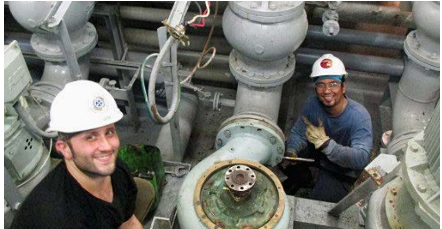
OVERSEAS SANTORINI 2nd A/E Emery Barg sent this one in of M.E.B.A. engineers fixing a seawater pump. The vessel was in the Strait of Malacca near the Philippines. At left is 1st A/E Vinny Quinones with 3rd A/E Arvie Viray.
